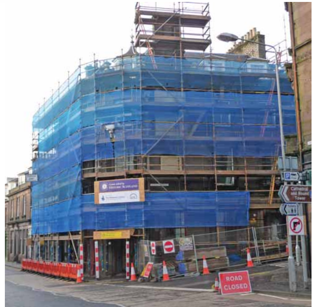
The restoration of the Dalhousie Bar building in Brechin is under way
