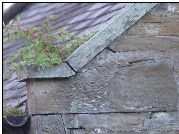
Holes in stonework
