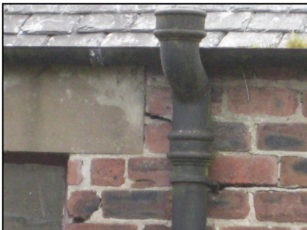
Spaces in brickwork
