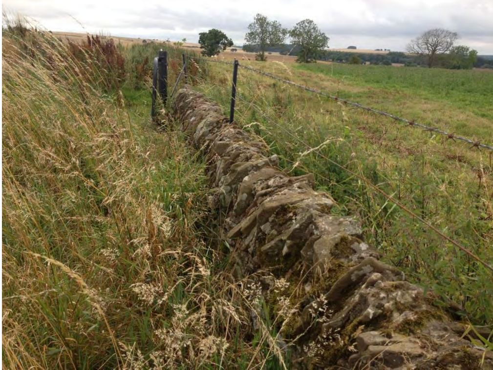
Photograph 7: A view of one of the stone wall boundaries in the west of the site.
