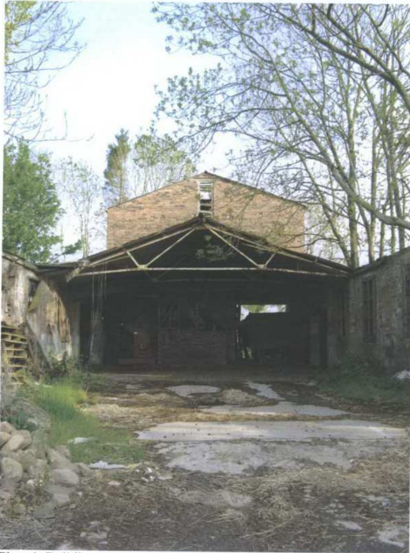
Plate 1. Buildings on the site were essentially unsuitable for bat roosting. The high ganery had no roof lining and no wall cladding and thus no potential roost sites. Other buildings were low, in very poor condition and with very few suitable roost sites. Trees were mainly small, with no cavities usable by bats.
