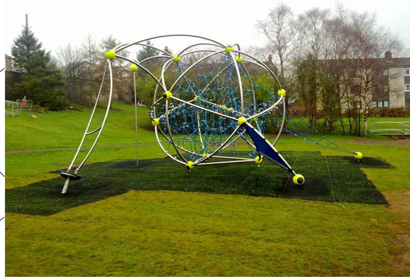
Supply and install 1 No Russell Leisure. Cosmo Spacenet Special, with duck jib, banister slide, climbing wall, fireman's pole, and access net. Supply and lay approx. 53m 2 of Safagrass safer surface. Supply and install 23 Nr green rubber safer surfacing tiles. Age range 5 to early teens
