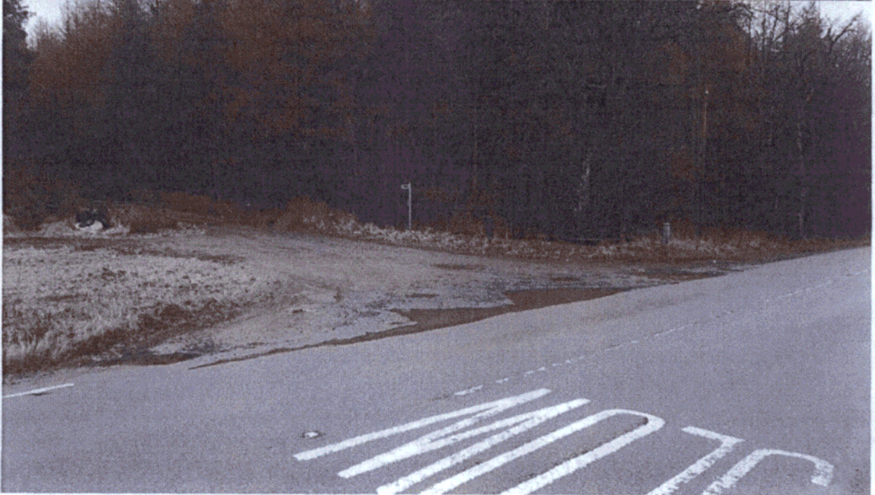
13. Junction of Checkbar road and A923. Incipient encroachment of lorry damage onto public highway
