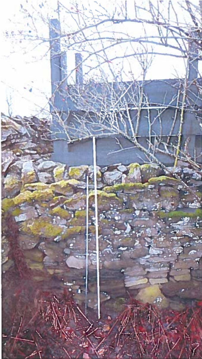
Photo 3 – Two canes are 5'-0" & 4'-0" high respectively. Discrepancy is that wall is detailed as 1.49M high (4'-10 5 / 8 " ) whereas it measures 1.32M (4'-4" ) on site – a discrepancy of 170mm.
