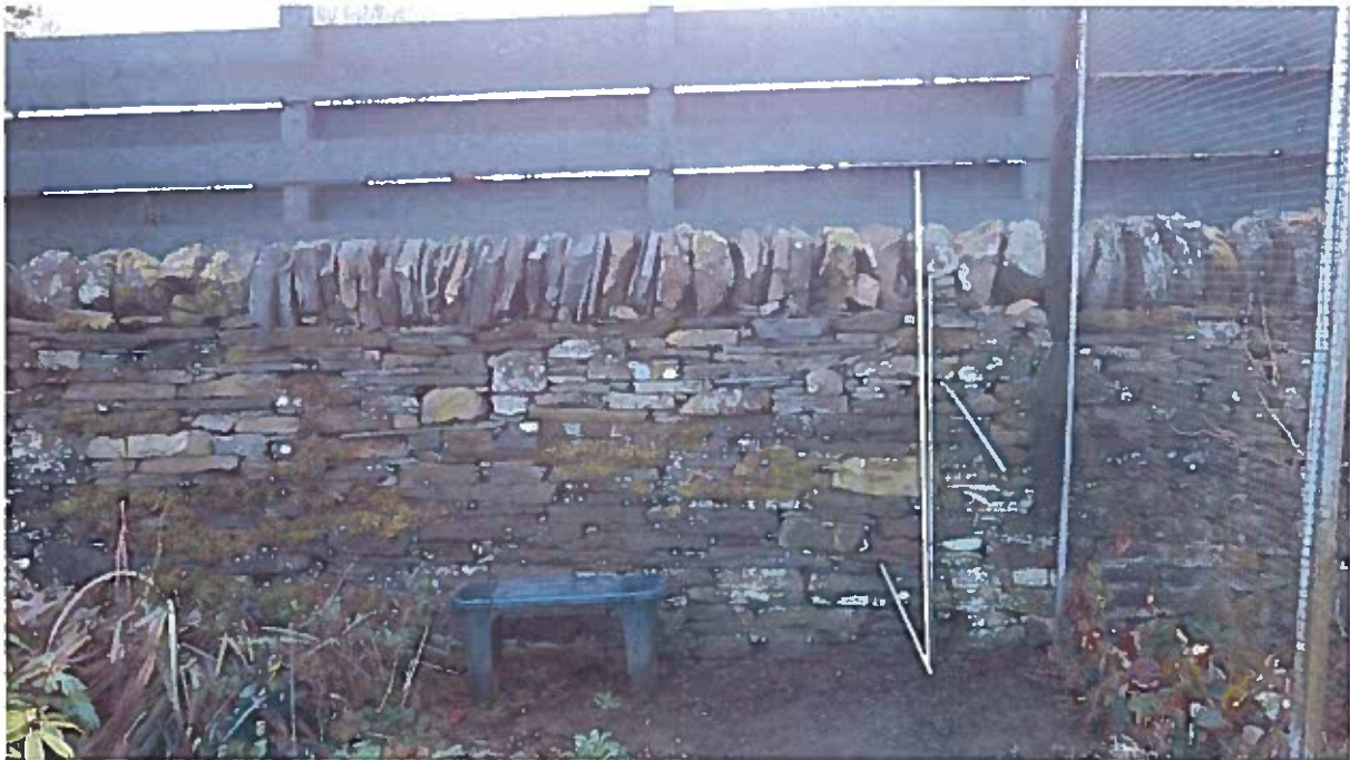
Photo 2 – Two canes are 5'-0" & 4'-0" high respectively. The two horizontal canes are the original ground levels and projected elevated ground levels respectively at Fern Cottage north boundary. Discrepancy is that wall is detailed as 1.5M (4'-11") whereas it measures 1.37M (4'-6") on site.
