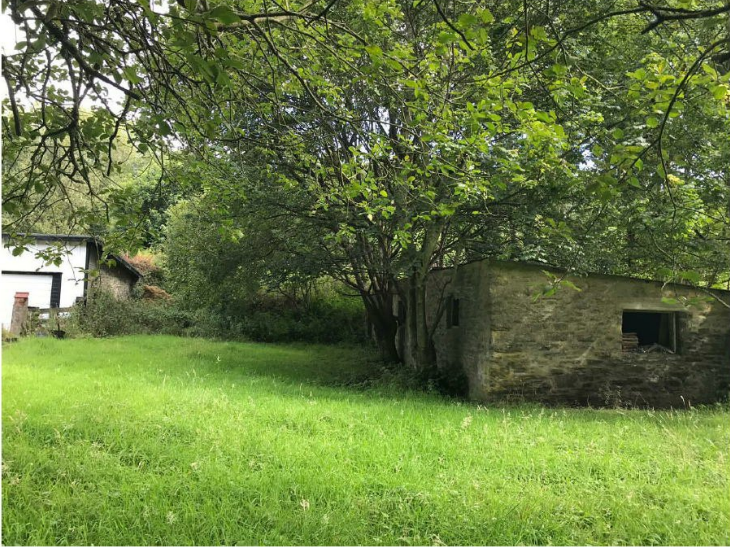
Figure 4: Dilapidated Bleach Works Building
