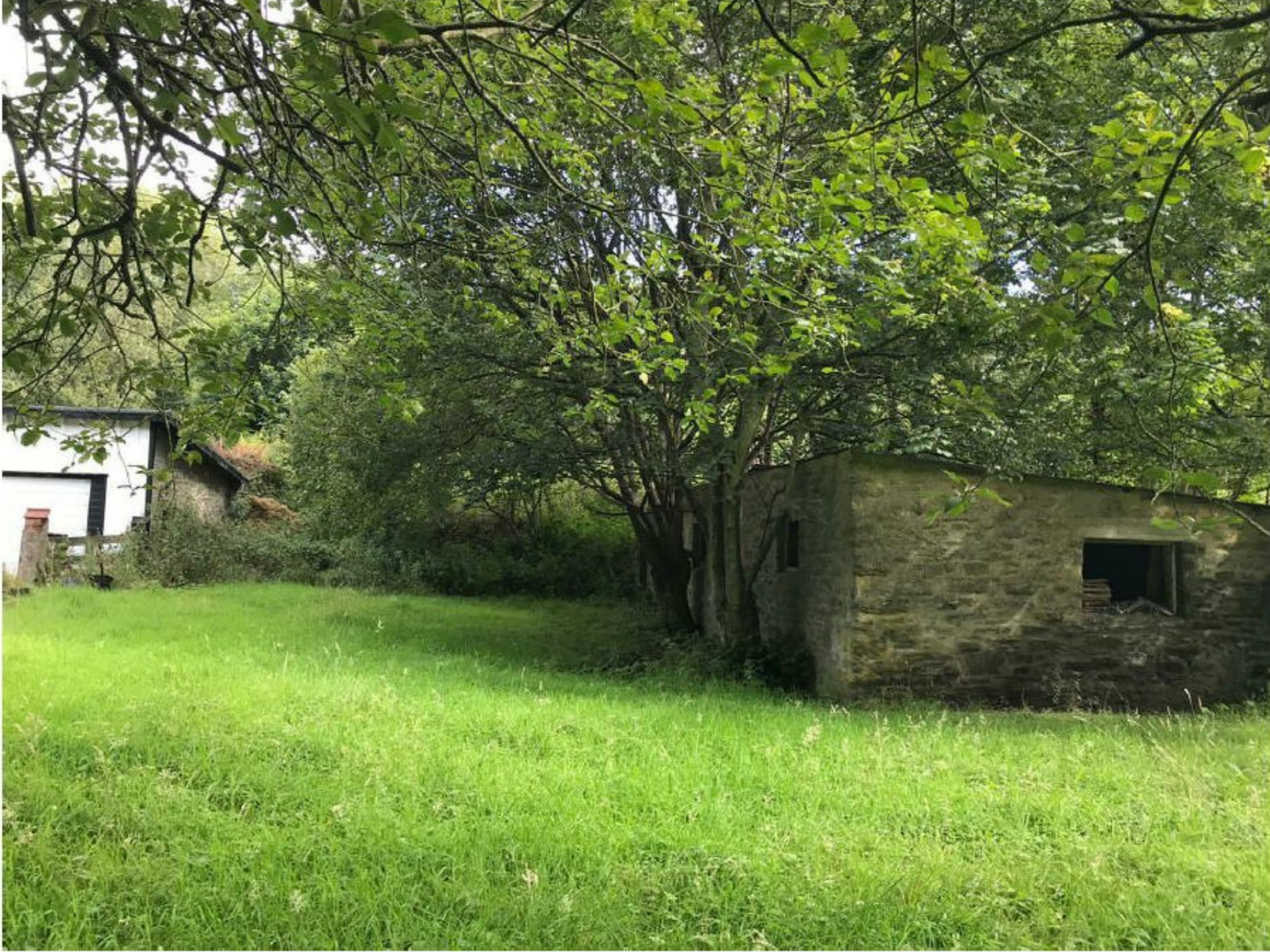
Figure 4: Dilapidated Bleach Works Building
