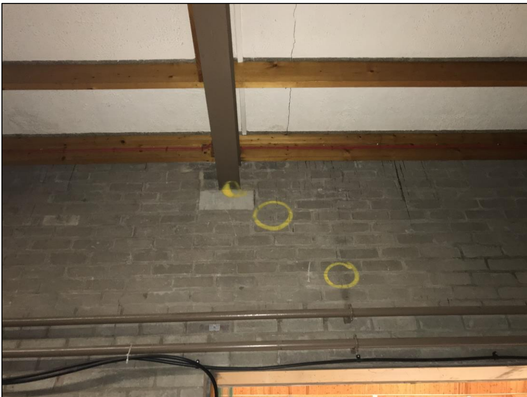
Figure 12 – Cracking Propagating Away from Padstone in Sports Hall Store
