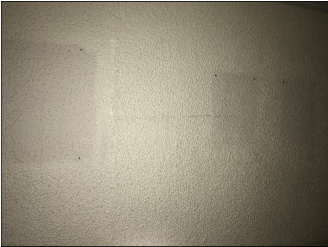
Figure 15 – Hairline Cracking on Finishes of Wall in Changing Room Corridor
