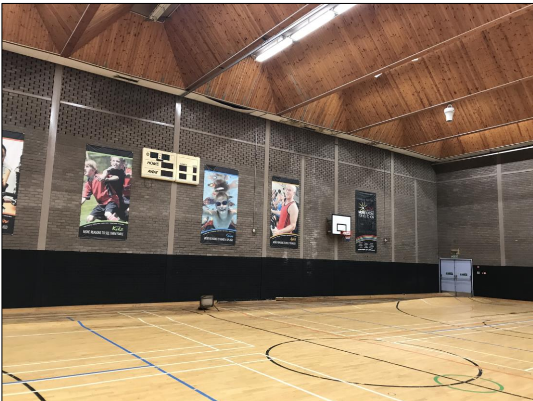
Figure 10 – Double Storey Sports Hall showing Water Ingress
