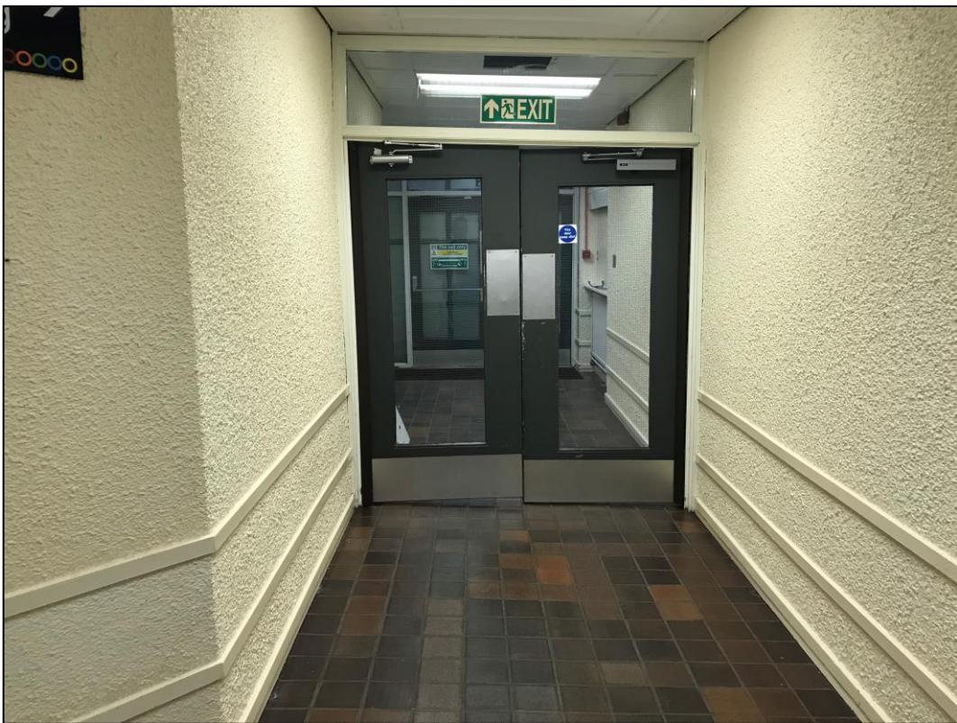
Figure 16 – Evidence of Floor Movement in Changing Room Corridor Area
