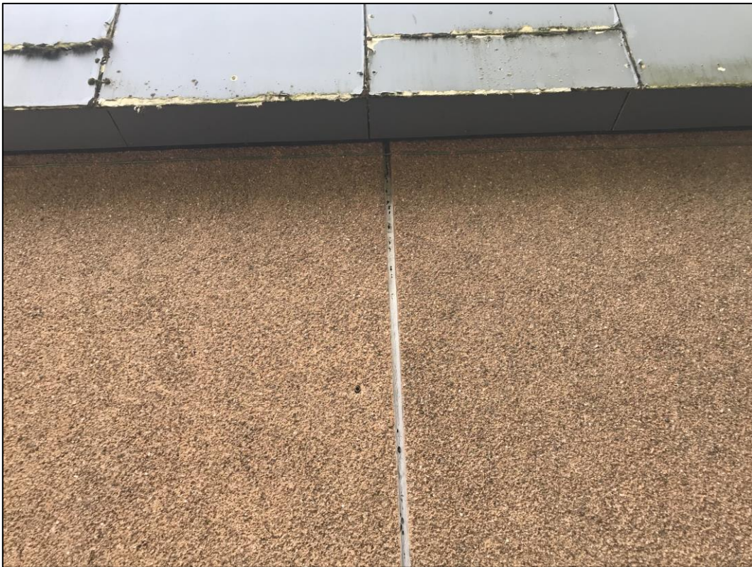
Figure 8 – Opening of Movement Joint on East Elevation
