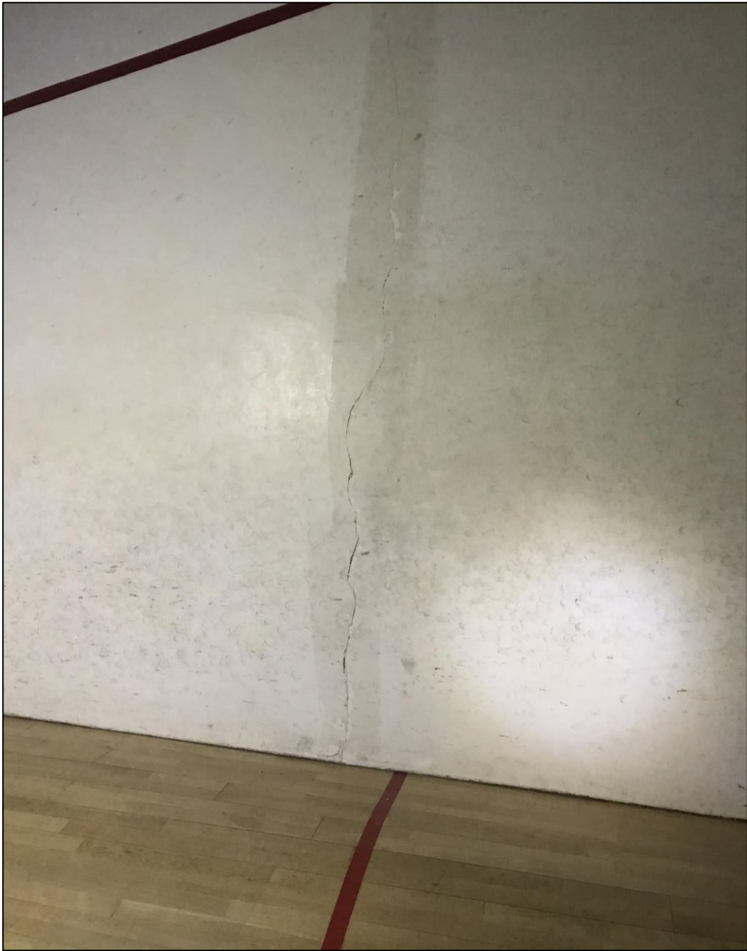
Figure 14 – Vertical Cracking on Finishes in Squash Court Area
