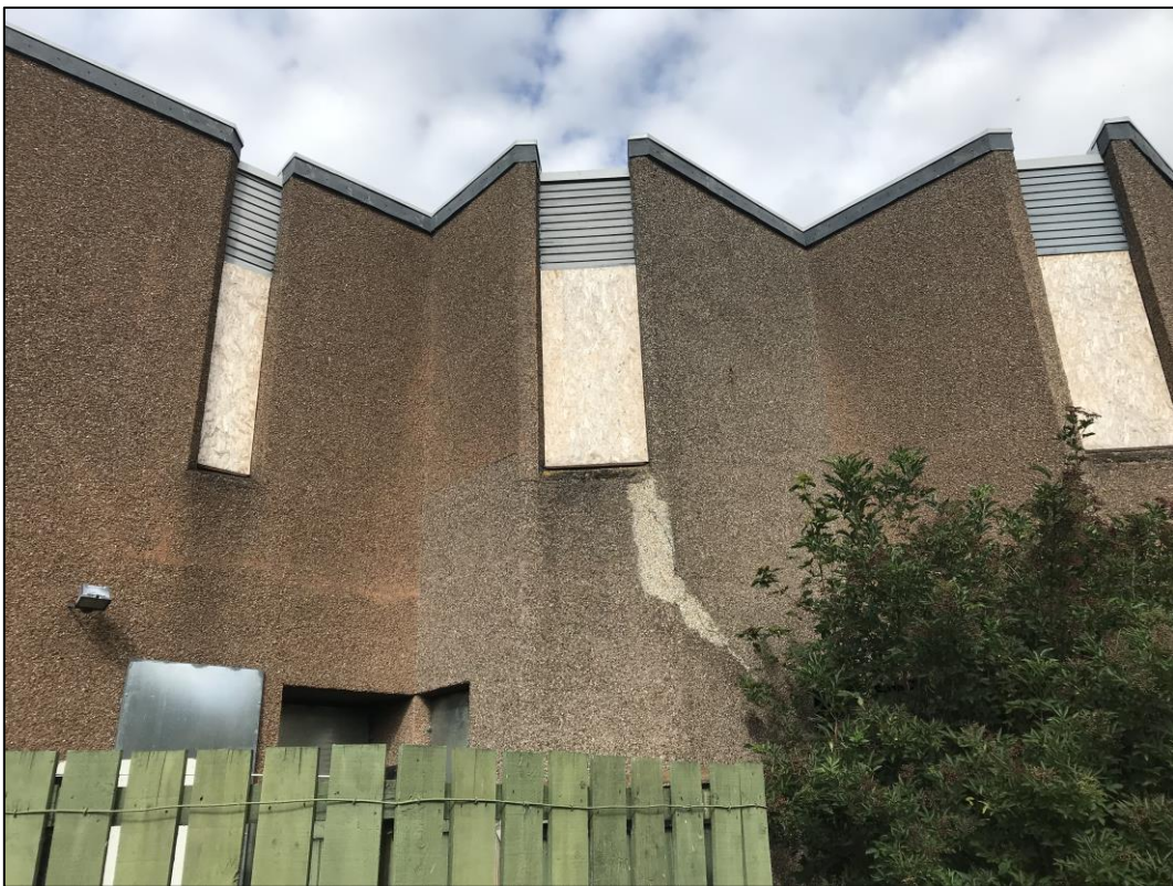
Figure 4 – Diagonal Cracking from Sill on South West Elevation
