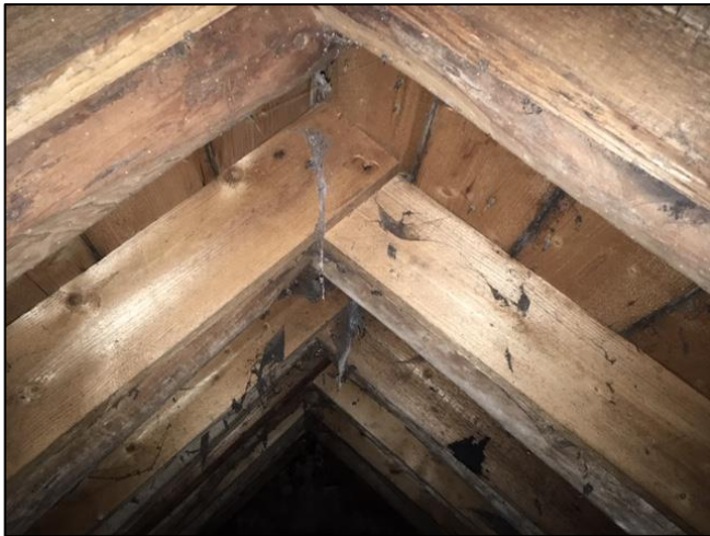
Photo 8: Cobwebbed sarking boards and apex inside bungalow
