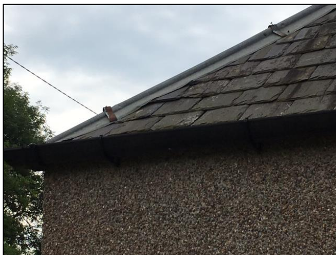
Photo 5: Typical gaps under ridge pieces in bungalow
