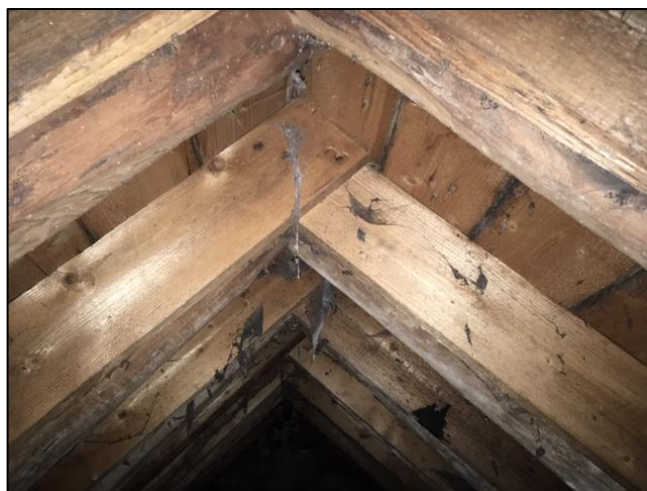
Photo 8: Cobwebbed sarking boards and apex inside bungalow
