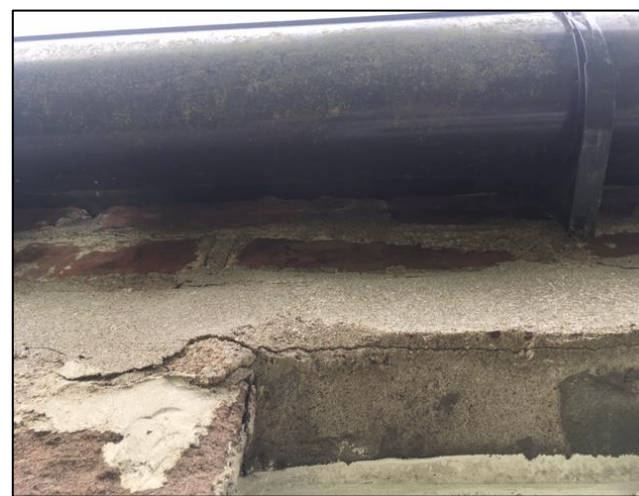
Photo 6: Gaps at wall head of bungalow under guttering
