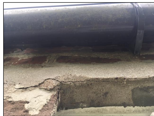
Photo 6: Gaps at wall head of bungalow under guttering
