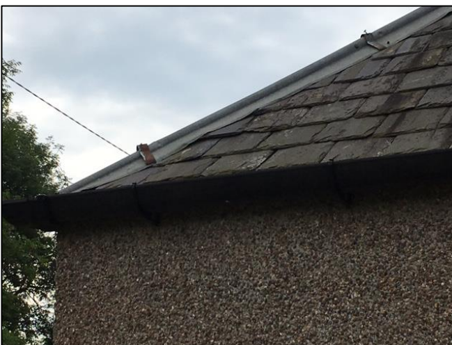
Photo 5: Typical gaps under ridge pieces in bungalow
