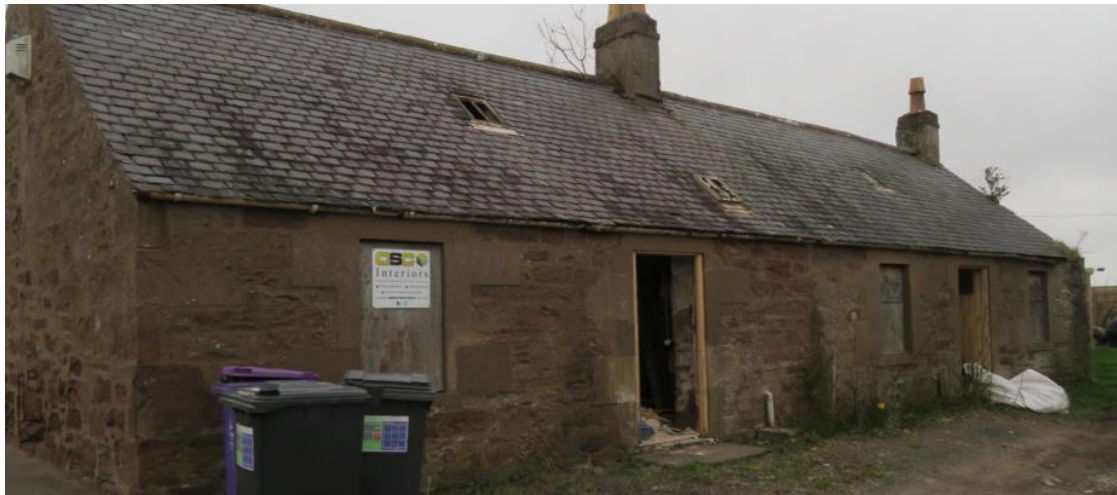
The derelict cottages on the site of No. 32 that have remained unaddressed through three owners.
