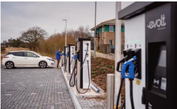
Image showing electric vehicle charging points at Orchardbank in Forfar.
