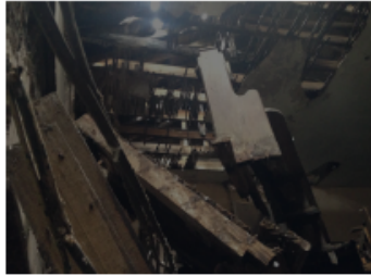
FIRST FLOOR ROTTEN
