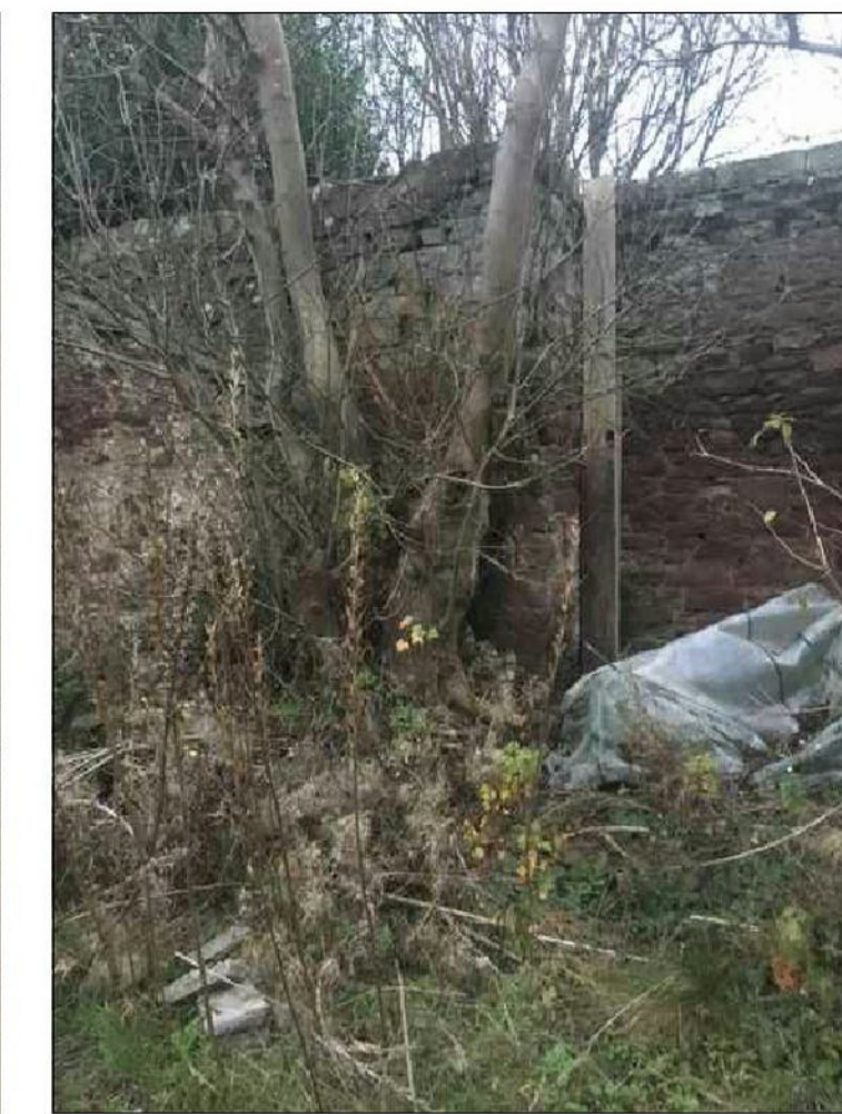
Rubbish littering the site
