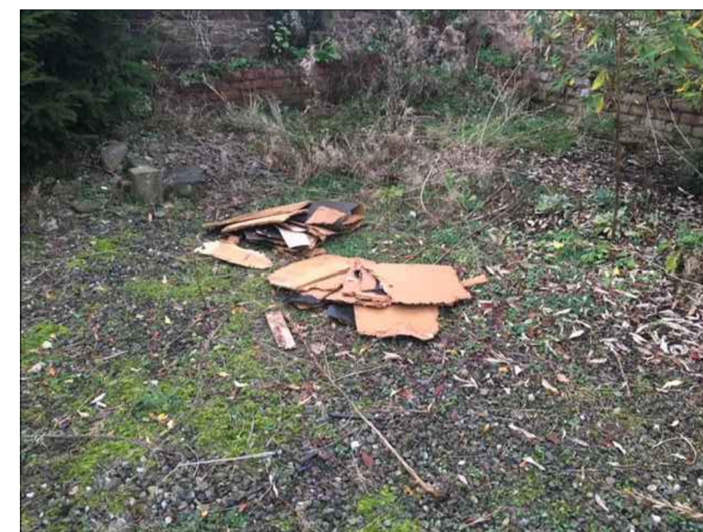
Rubbish left on site
