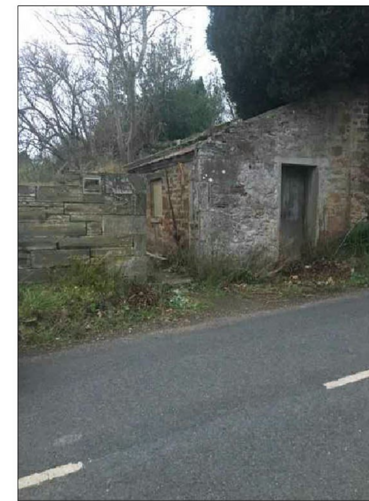
Existing store and gable end of former Church Hall forming site boundary.
