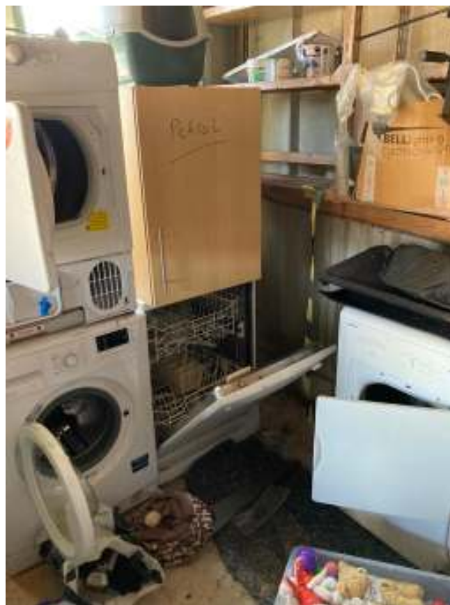
Image showing existing commercial white goods servicing the cattery
