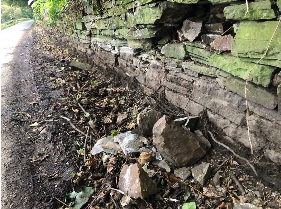
Figure 6: The damage to the stone dyke.
