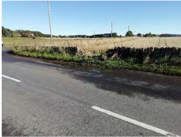
Figure 2 : Distant view of damage to dry stone wall
