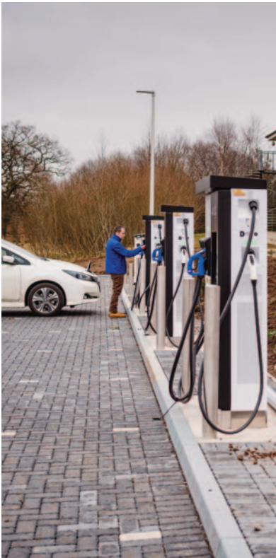
Image showing electric vehicle charging points at Orchardbank in Forfar.
