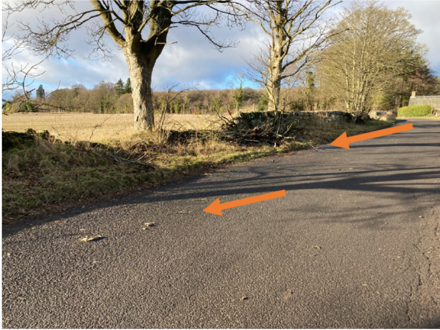
Fallen vegetation and branches on the road
