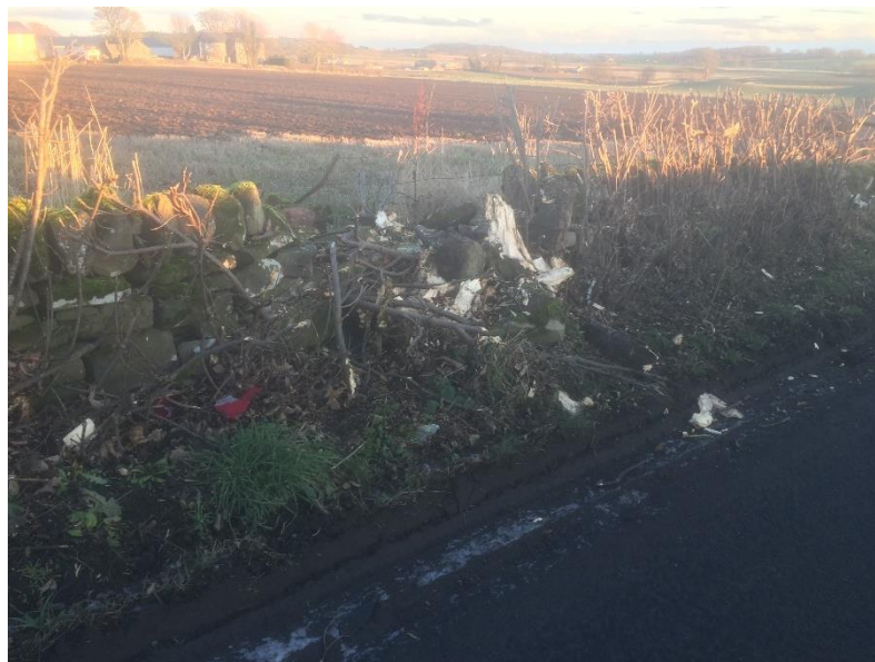
Picture of stoved dyke, accident 02/01/21
