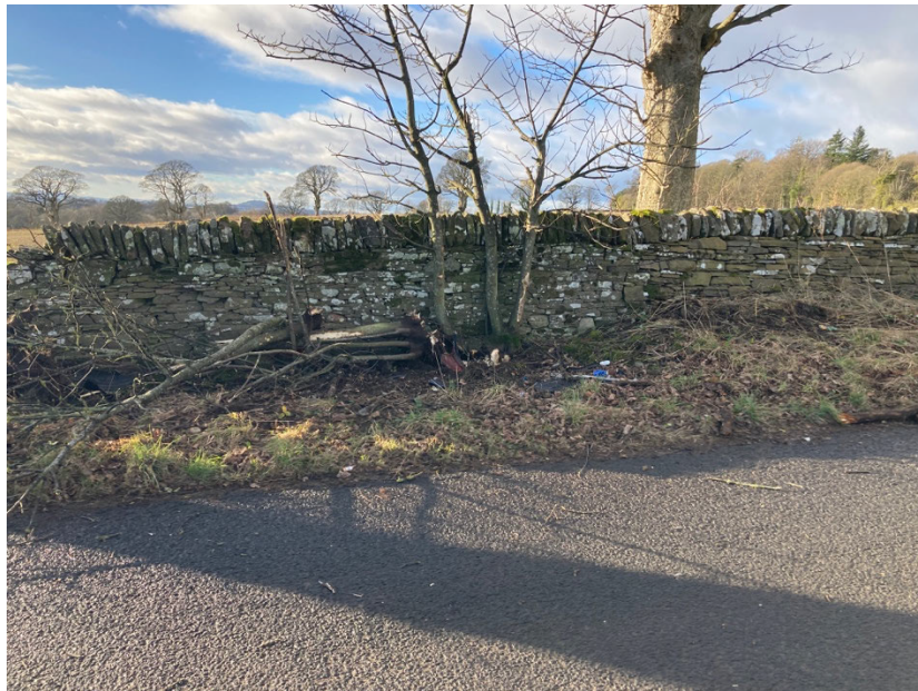
Distant view of damage to vegetation
