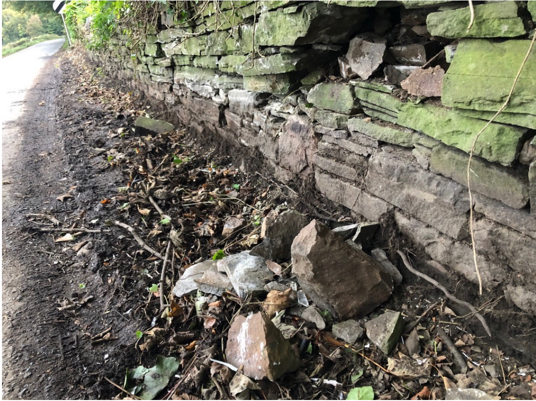
Figure 6: The damage to the stone dyke.
