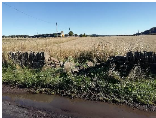
Figure 1 : Close up view of damage to dry stone wall
