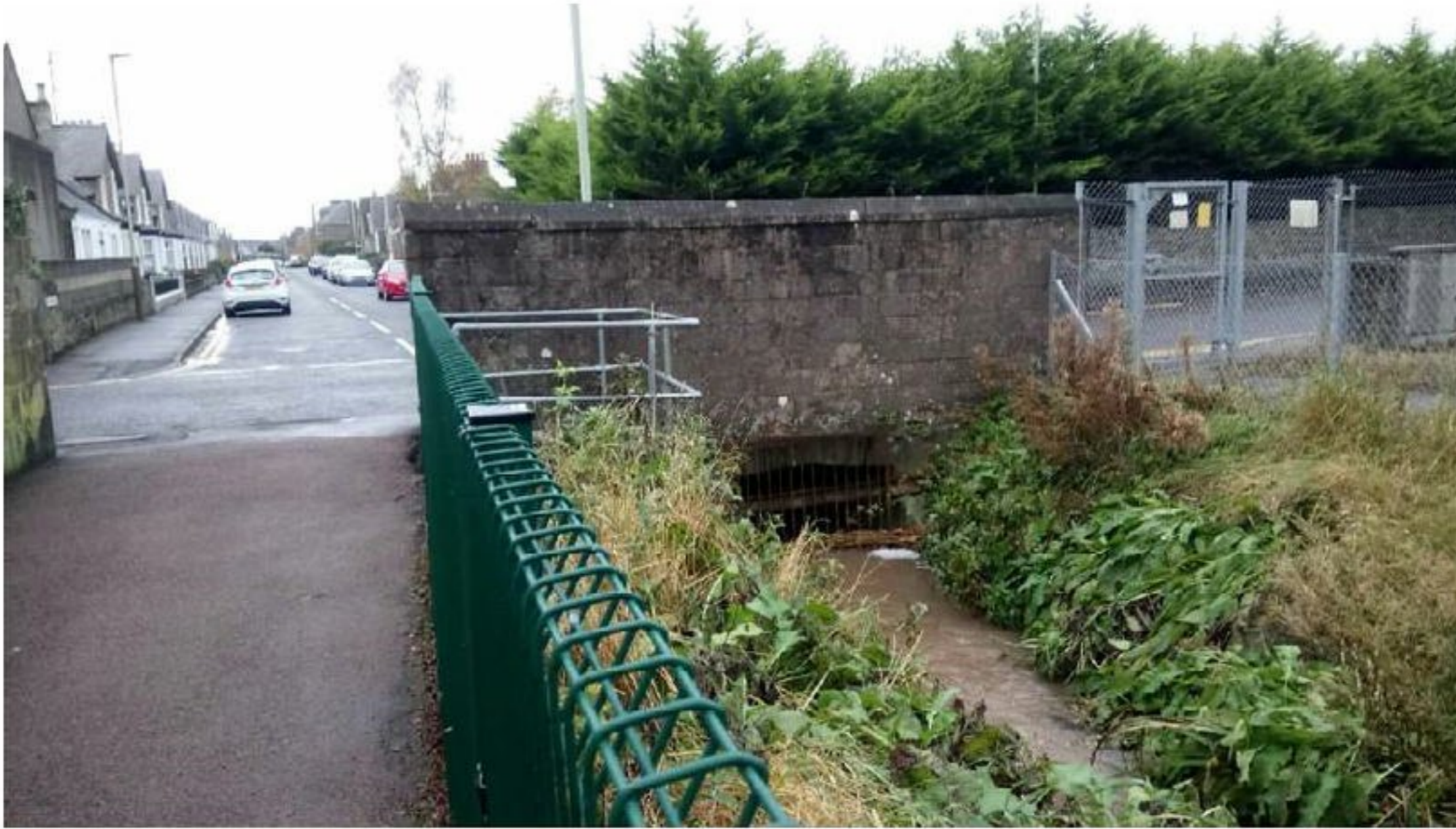
Photograph 2 – A view of the Monifieth Burn culvert which runs past the site, at its upstream end at Ramsay Street.
