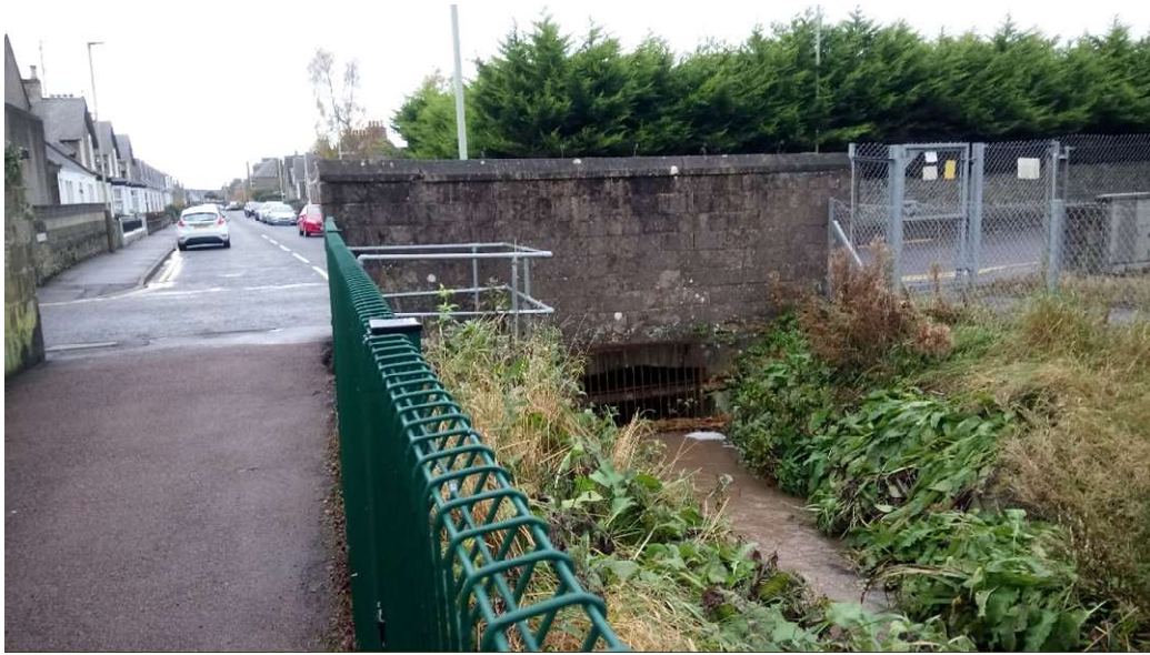
Photograph 2 – A view of the Monifieth Burn culvert which runs past the site, at its upstream end at Ramsay Street.
