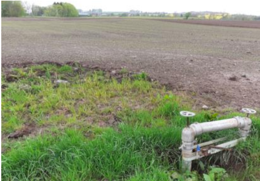
Top image: pipes, presumably some sort of water management / irrigation system installed by the applicant; source and destination of water unknown
