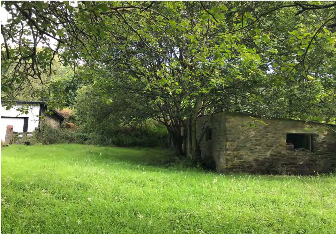
Figure 4: Dilapidated Bleach Works Building
