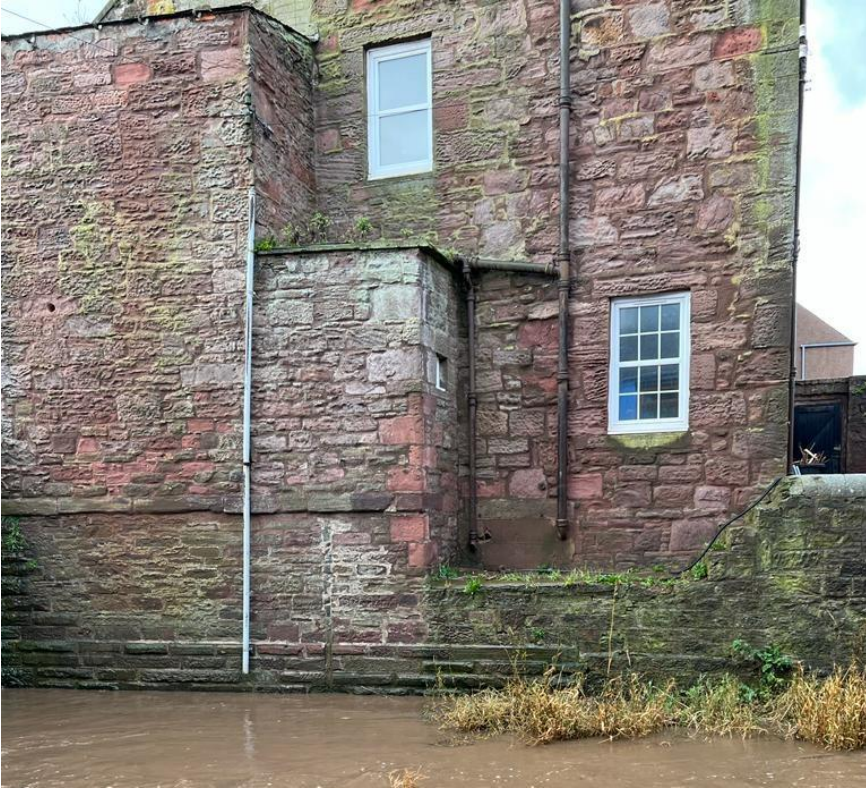
PHOTO A – taken in March 2023 after continual heavy rainfall. Water level approx. 3.000m
