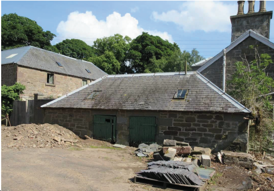
Photo 17. Building O (the buildings to the right and left are not within the site).
