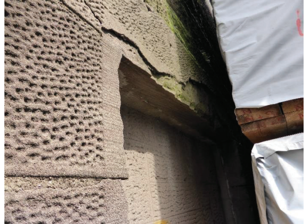
166 Cracked + spalling lintel
