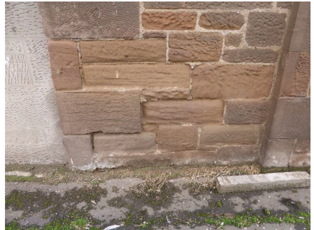
71 Stone decay + open joints
