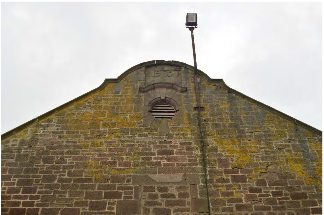
Illus 9 Detail of circular vent, hoodmould and build date on the SW façade.
