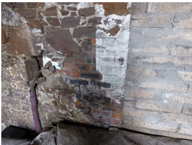
31 Crude repairs + hole through wall
