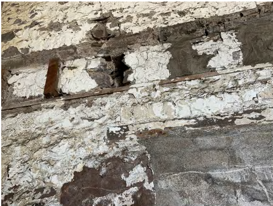
Figure 22: Internal North East Elevation –Intermediate Floor, Patches & Cracking
