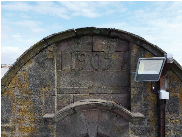
20 Cracked + delaminating at ornate masonry
