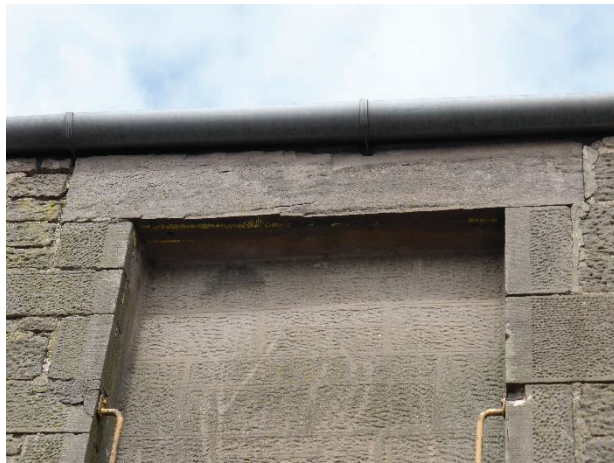
180 Cracked + spalling lintel + cracked rybats
