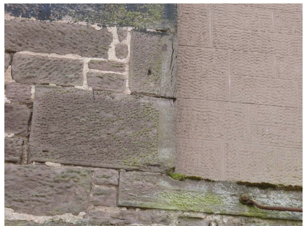
111 Cracking at rybats
