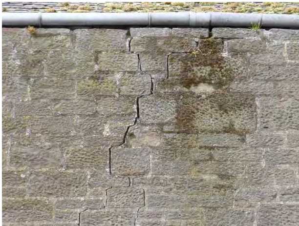
154 Structural movement cracks
