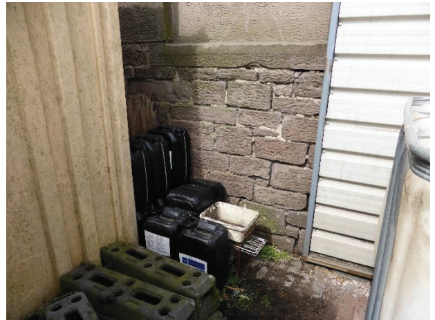
172 Failed pointing + open joints
