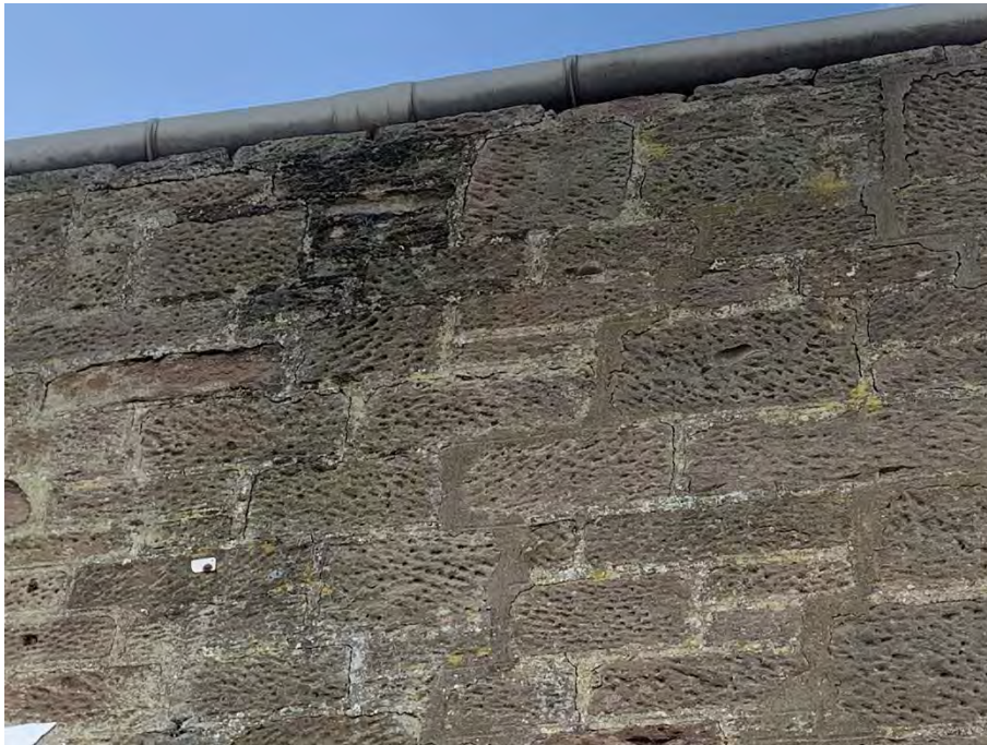
Figure 11: North East Elevation – Damp Patch, Weathered Stone ,Cracking & Gutter Position
