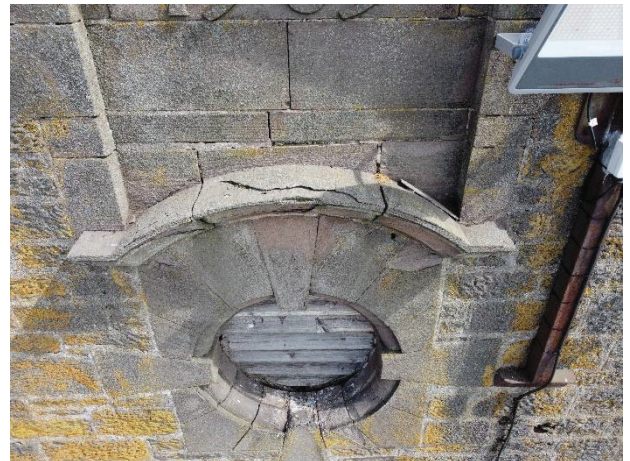
23 Cracked + delaminating at ornate masonry
