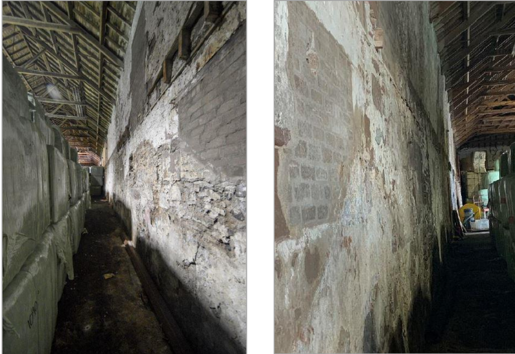
Figure 9: NW and NE facing interior walls – showing reduced storage capacity with goods kept away from the walls due to wall lean, patches and cracking
