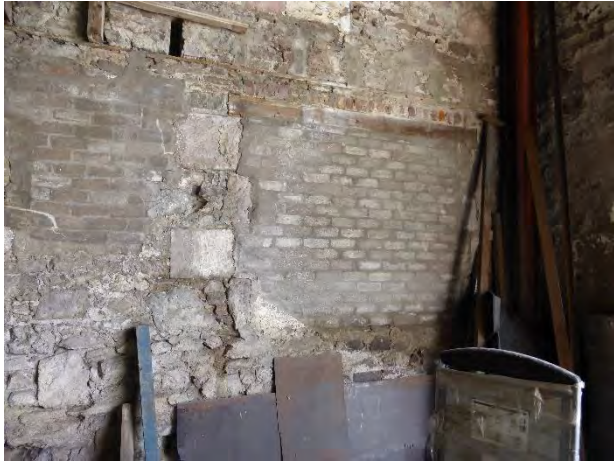
16 Crude repairs + pockets of missing rubble
