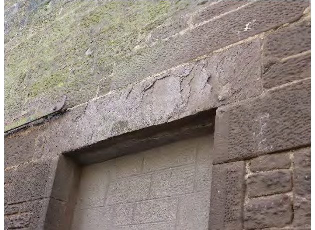
100 Spalling + cracking at lintel
