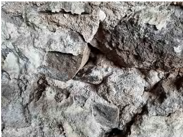
1 Loose + missing rubble
