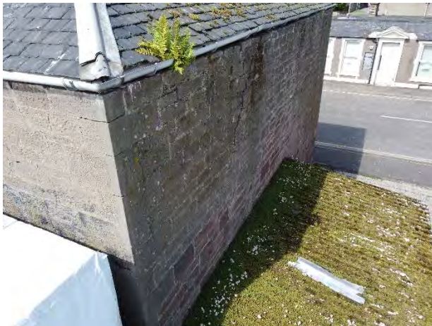
48 Outwards leaning of the wall
