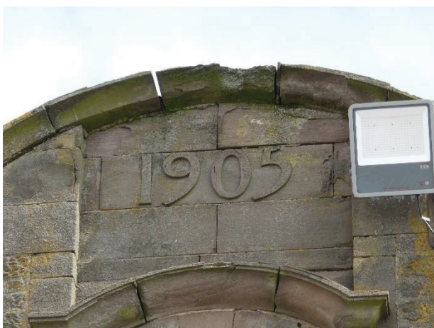
198 Cracked + delaminating at ornate masonry
