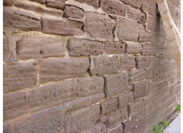
137 Stone decay + open joints
