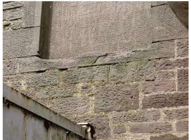
177 Delaminating + spalling sill
