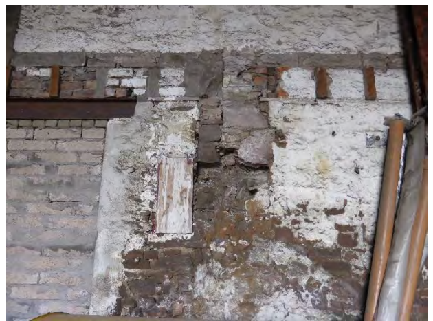
29 Crude repairs + pockets of missing rubble
