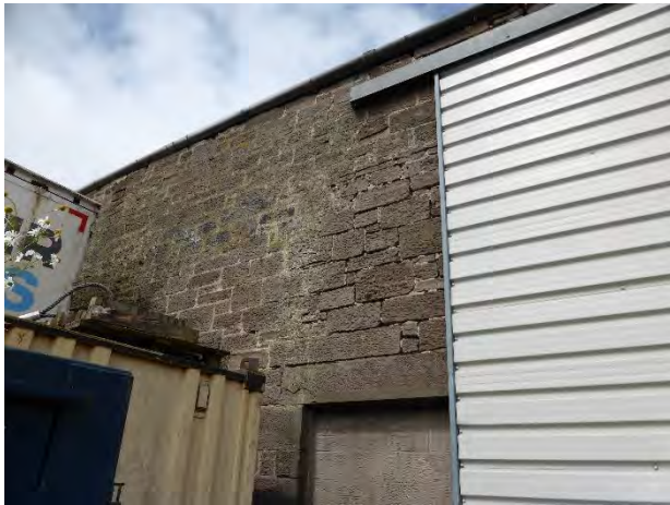
171 Failed pointing + open joints
