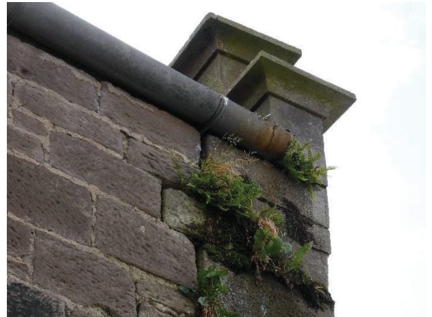
Structural movement + widened joints
