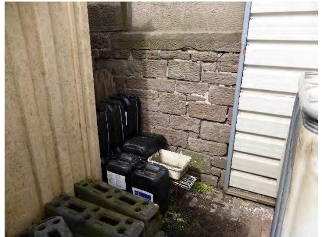
172 Failed pointing + open joints
