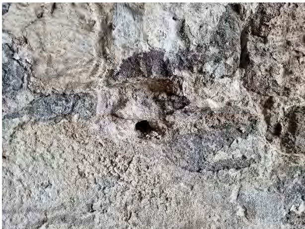
2 Loose + missing rubble
