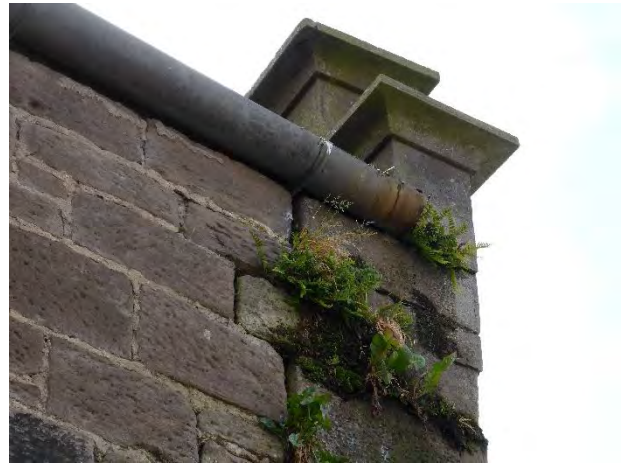
Structural movement + widened joints
