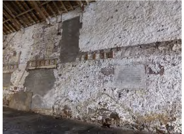
19 Crude repairs + pockets of missing rubble
