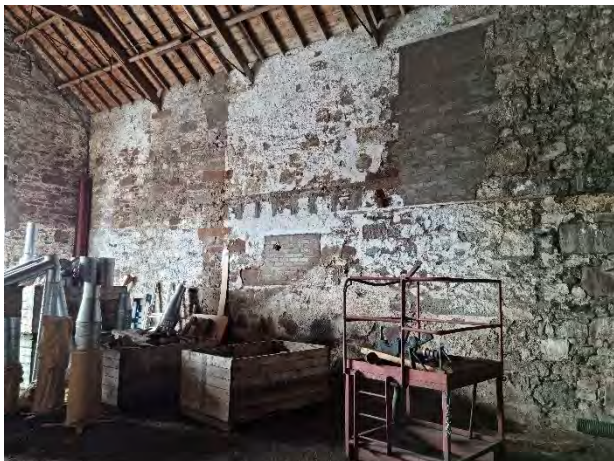
6 Crude repairs + pockets of missing rubble
