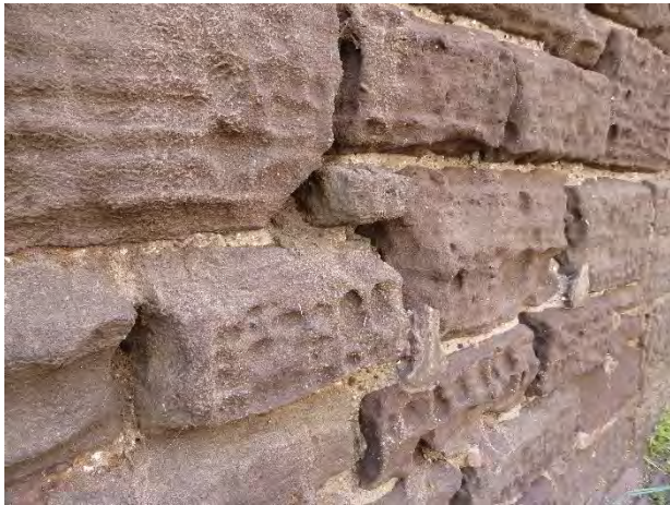
138 Stone decay + open joints
