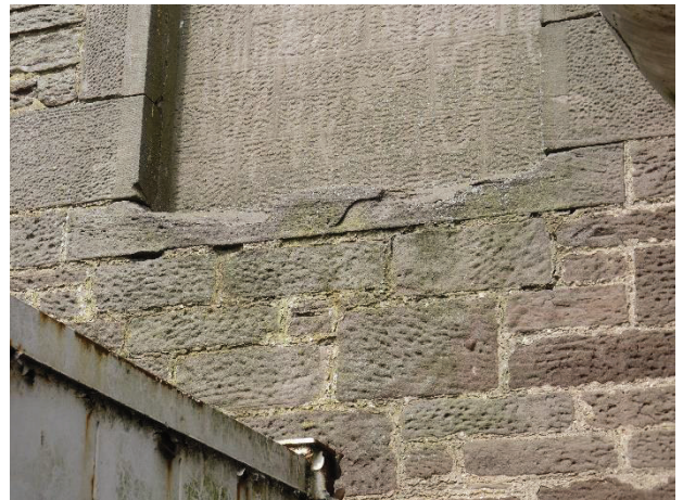
177 Delaminating + spalling sill
