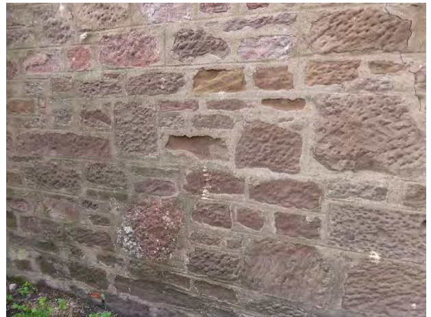
156 Cement mortars + stone decay
