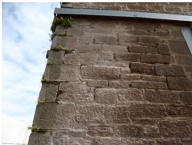
209 Stone decay + open joints + vegetation
