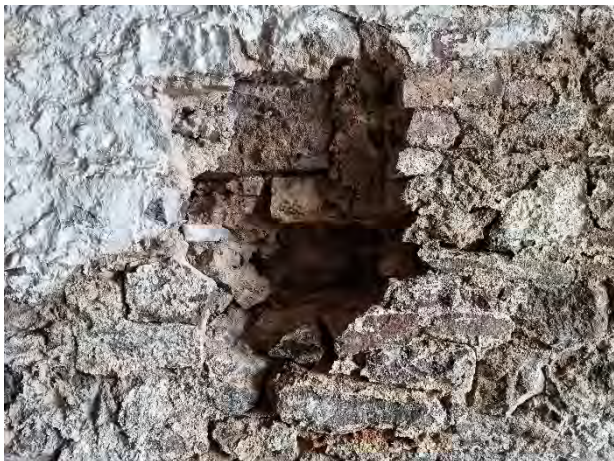
4 Loose + missing rubble
