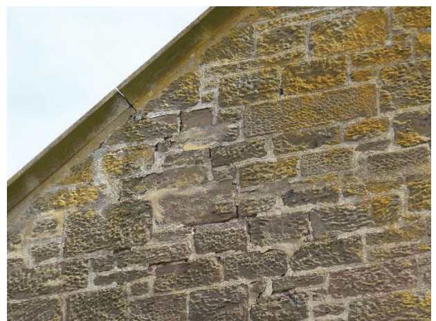
200 Stone decay + open joints
