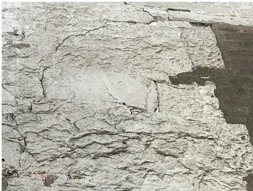
Figure 23: Internal North East Elevation –Diagonal Crack
