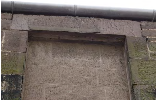
91 Spalling + cracking at lintel
