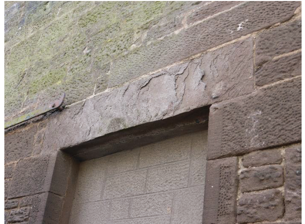
100 Spalling + cracking at lintel
