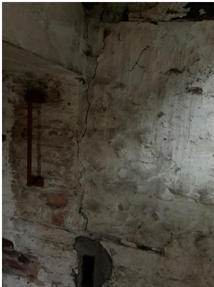
Photograph 3.21 - Old Workshop/Store –California Street Wall Crack
