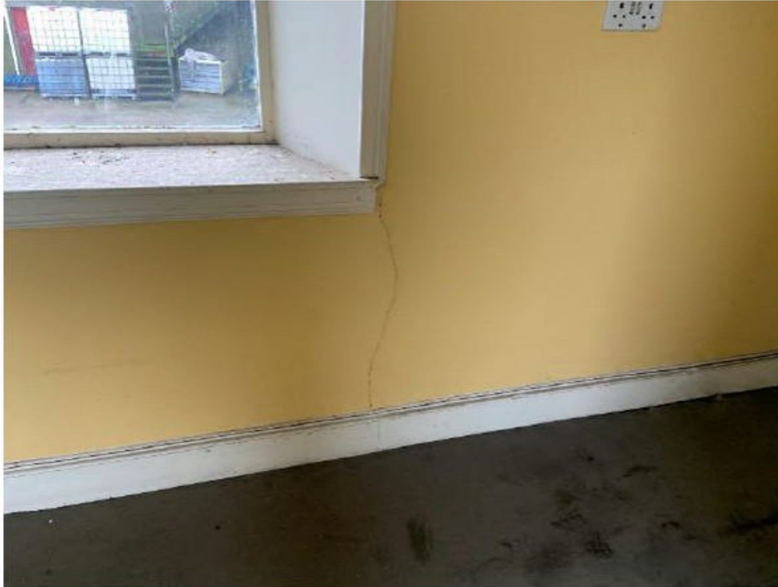
Photograph 2.14 America Street Offices – Internal - Cracks
