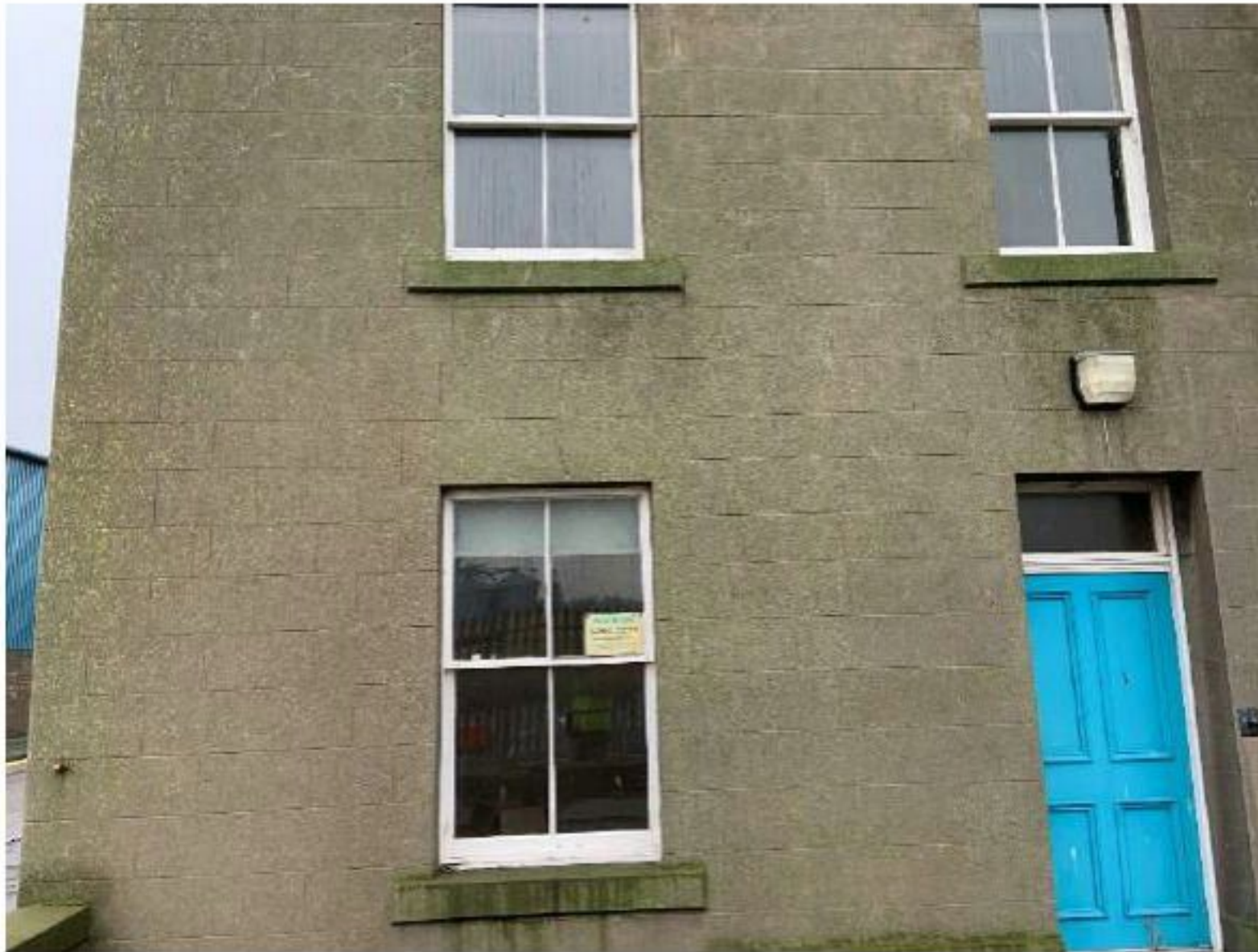
Photograph 1.02 Managers House - External Wall - Crack 1
