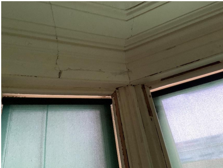
Photograph 1.11 Managers House - Internal Wall – Bay Window Cracking
