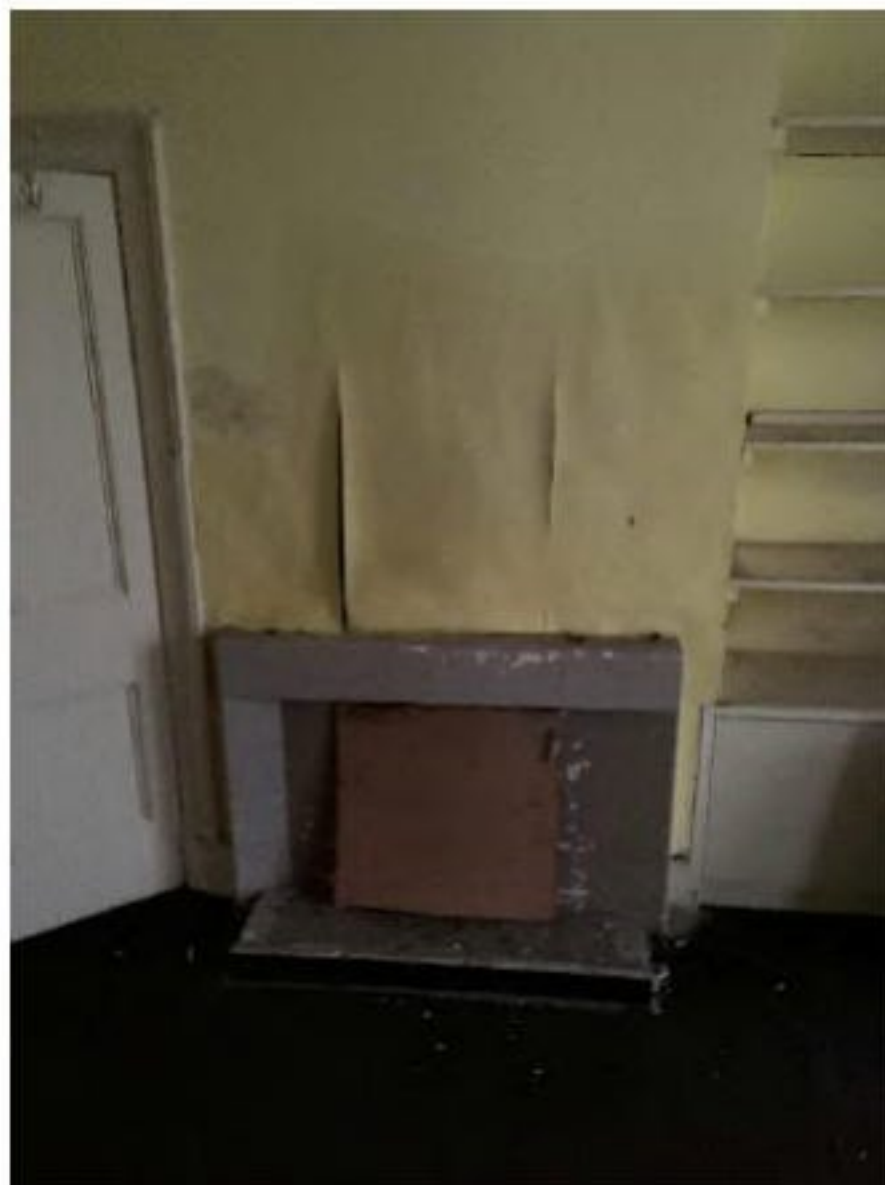
Photograph 1.09 Managers House - Internal Wall Fireplace & Dampness
