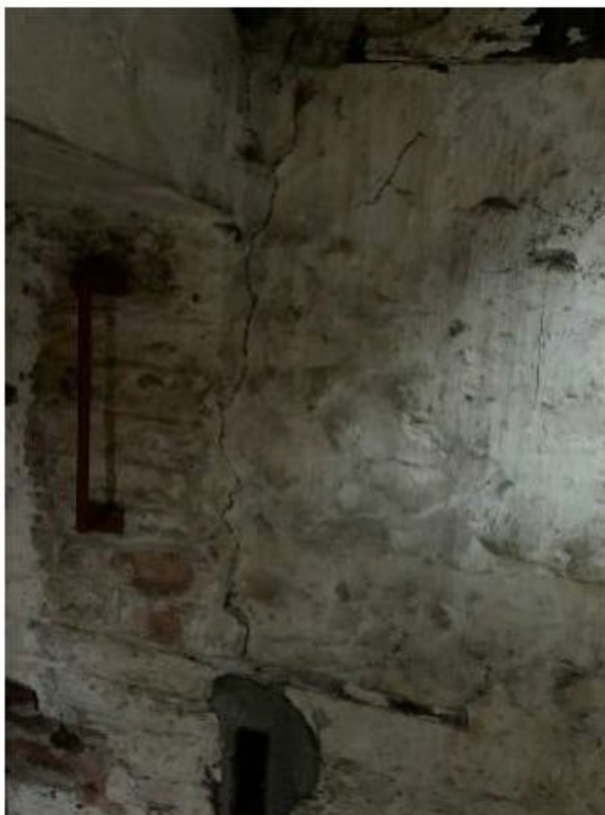
Photograph 3.21 - Old Workshop/Store –California Street Wall Crack
