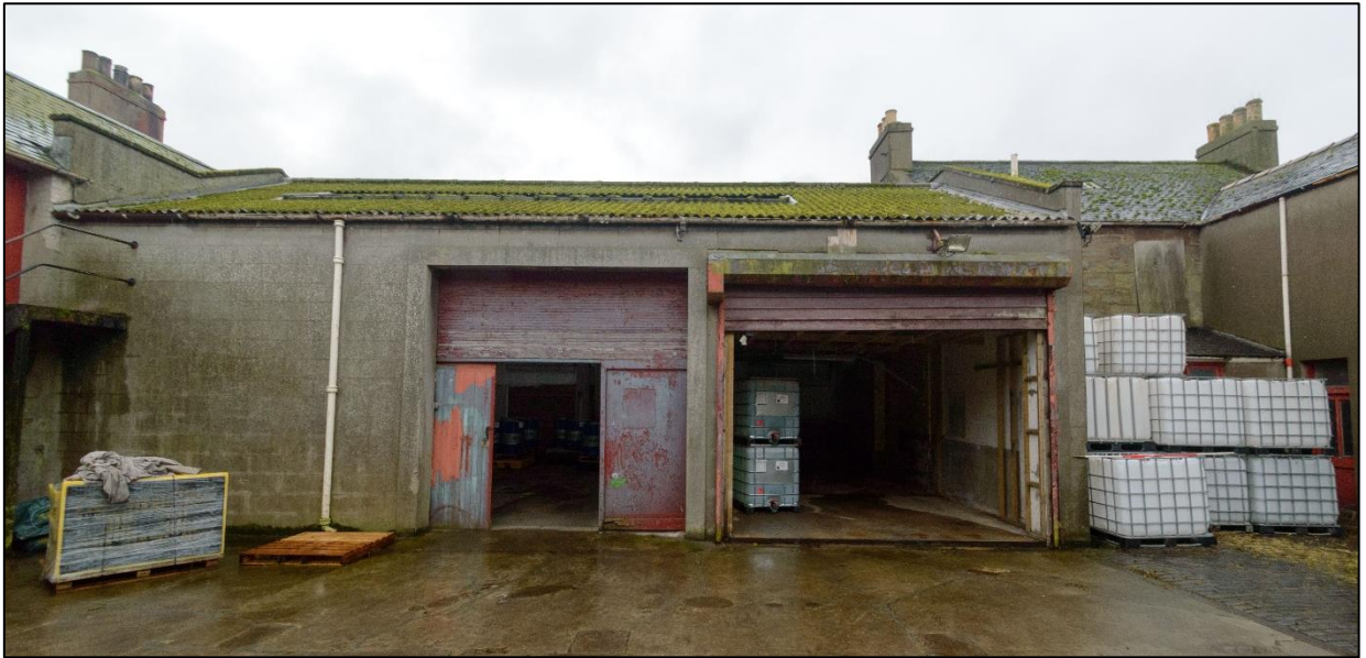
Illus 14 The SW courtyard elevation comprising the substantial garage or warehouse extension (room 10).
