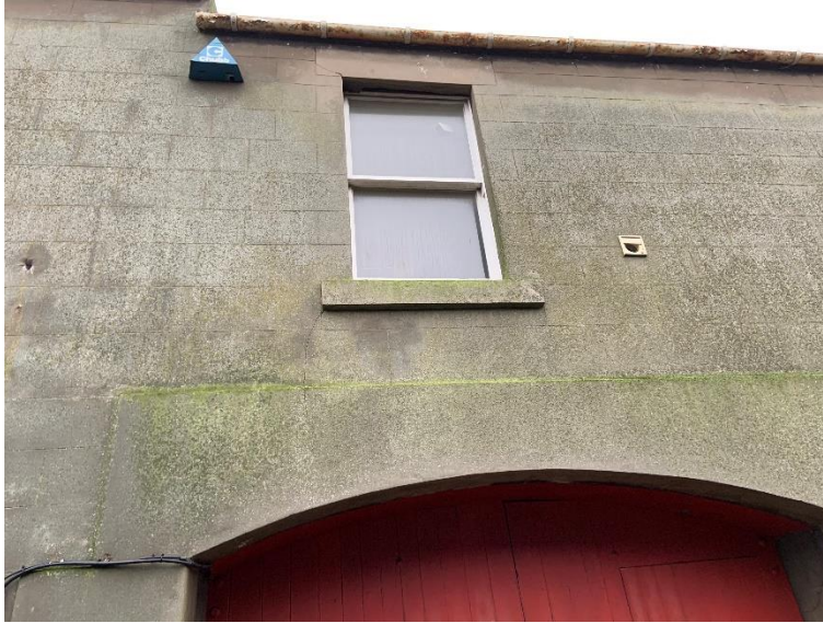
Photograph 2.04 America Street Offices - External Elevation – Crack at Arch
