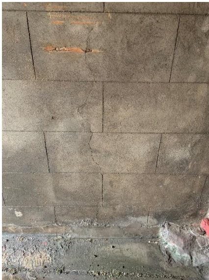
Photograph 2.05 America Street Offices - External Elevation – Crack in Archway
