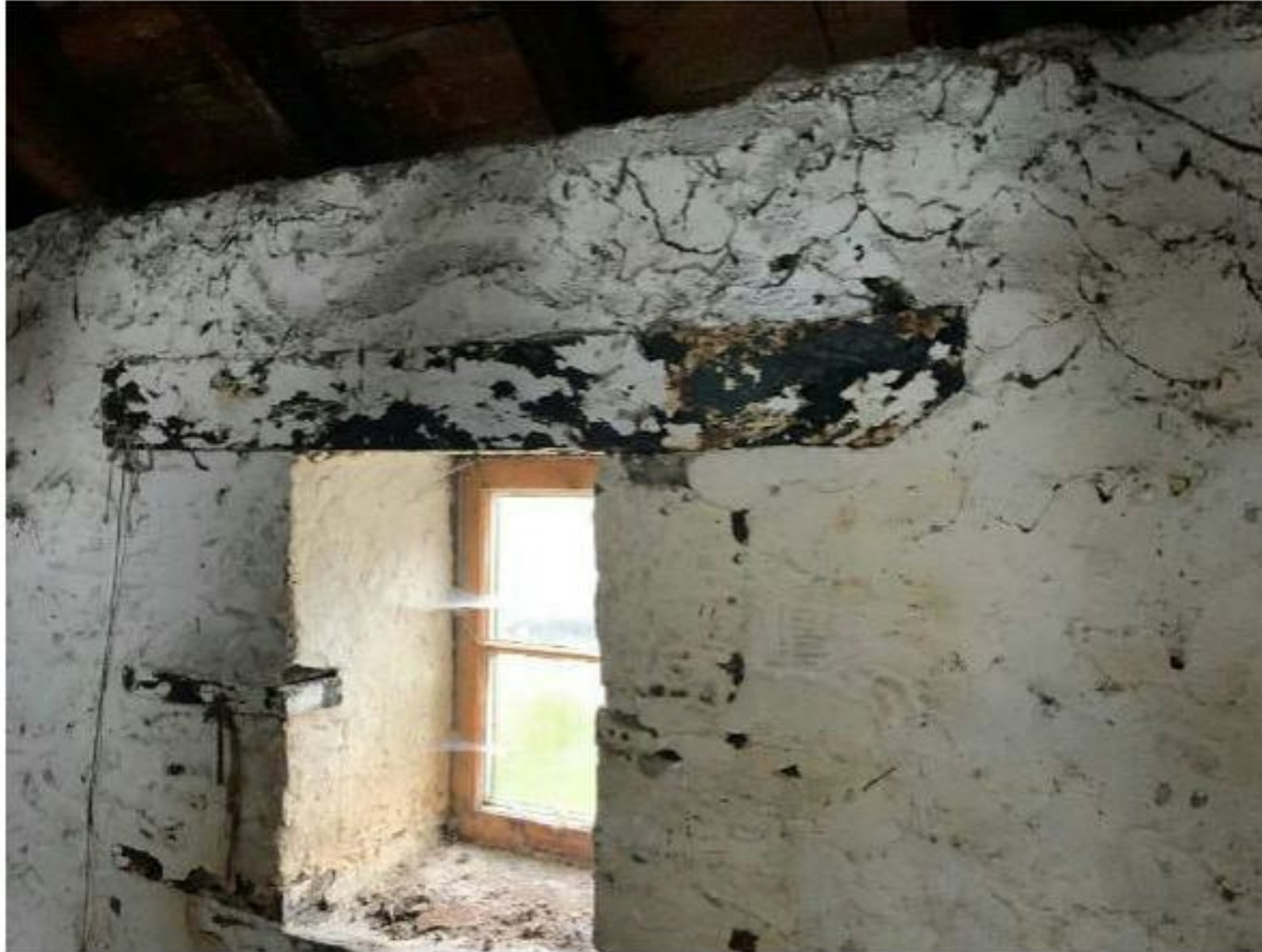
Photograph 3.22 - Old Workshop/Store –California Street Wall Lintel
