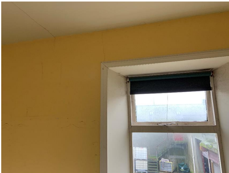
Photograph 2.13 America Street Offices – Internal - Cracks
