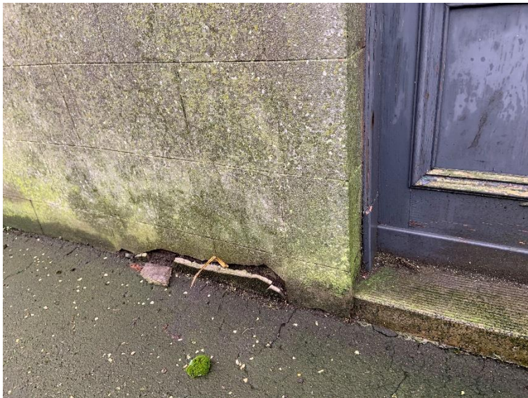
Photograph 2.03 America Street Offices - External Elevation – Base Render Spalling
