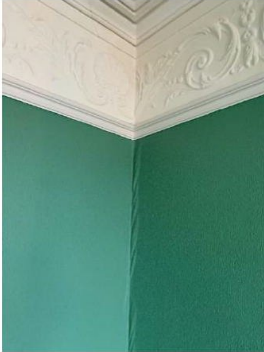
Photograph 1.10 Managers House - Internal Wall - Settlement
